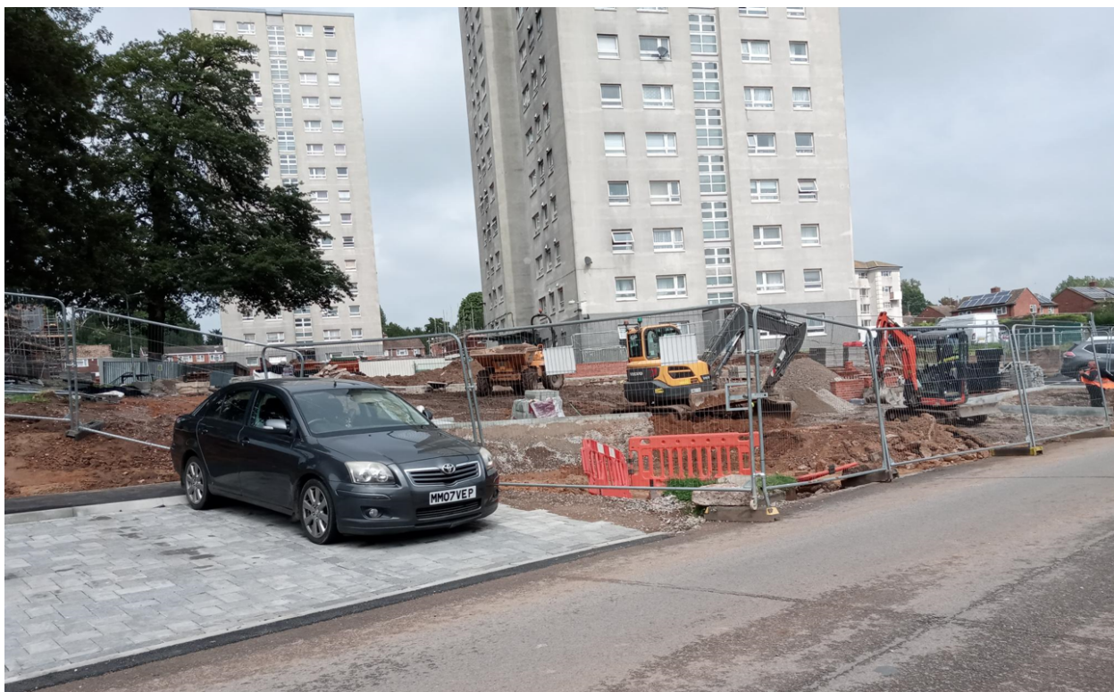
Figure 5 – Ongoing construction works, showing Wensley Court (background) and Riversley Court (right). Irving Court is not in photo (further to the left) (18/08/2023)
